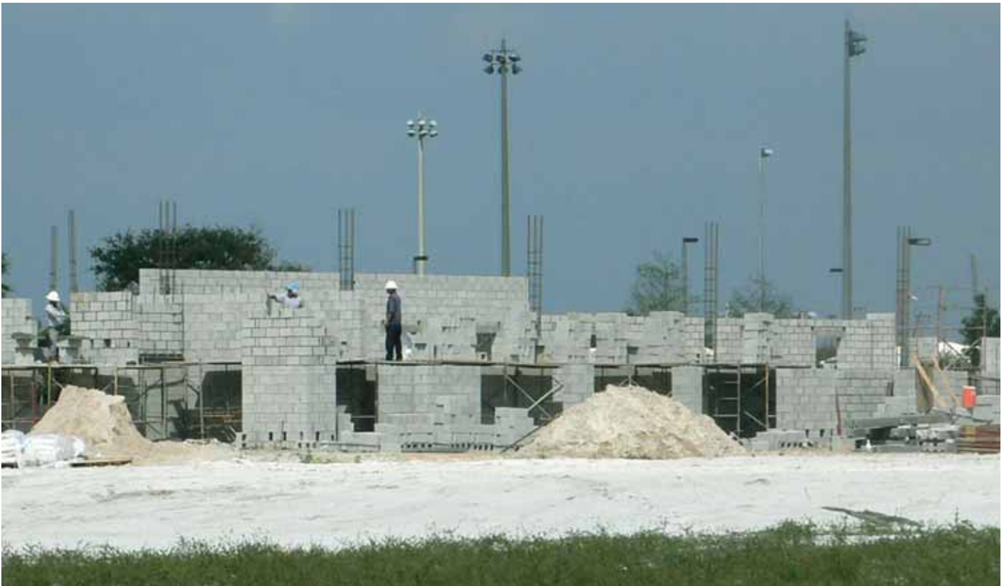
Construction is underway of the first two story 20,000 sq.ft. building in Phase I at our Professional Center at Wellington project in Palm Beach County.
